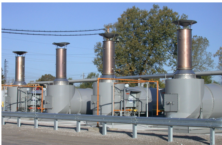
Four thermal oxidizers on the refinery property are being used to burn the vapors piped from the system of extraction wells.
