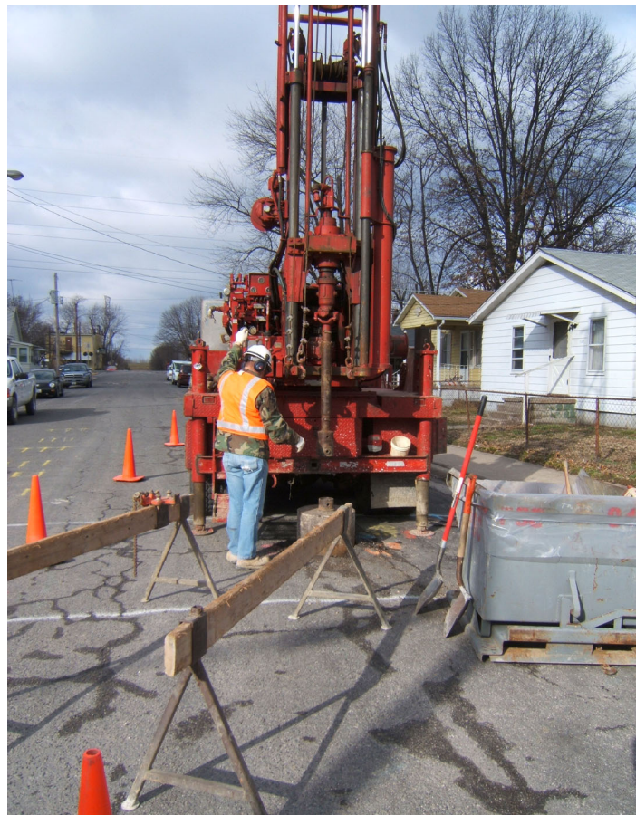
Drill rigs like this one will be used to install the additional SVE wells.
