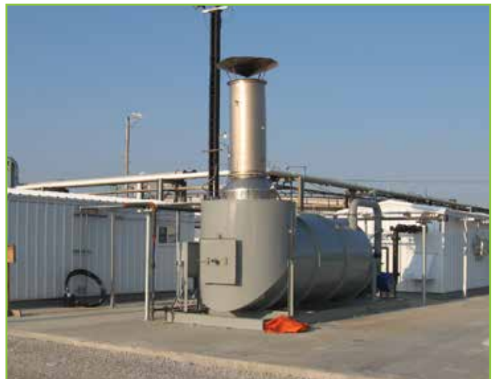
Thermal accelerator treating vapor from a refinery soil remediation project.
