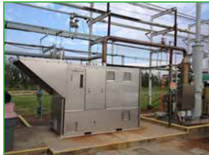
Chlorinated Catox with HCL scrubber
