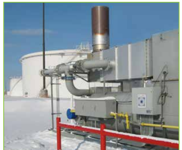
Thermal oxidizer installed at a petroleum distribution facility. The modular unit features heat exchange, heat exchange by-pass and catalyst module.
