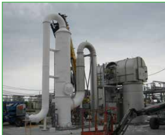
RTO with HCL Wet Scrubber
